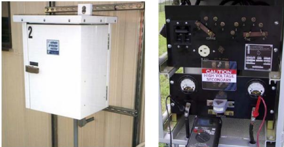
Figure 3 – Typical ICCP Rectifier
